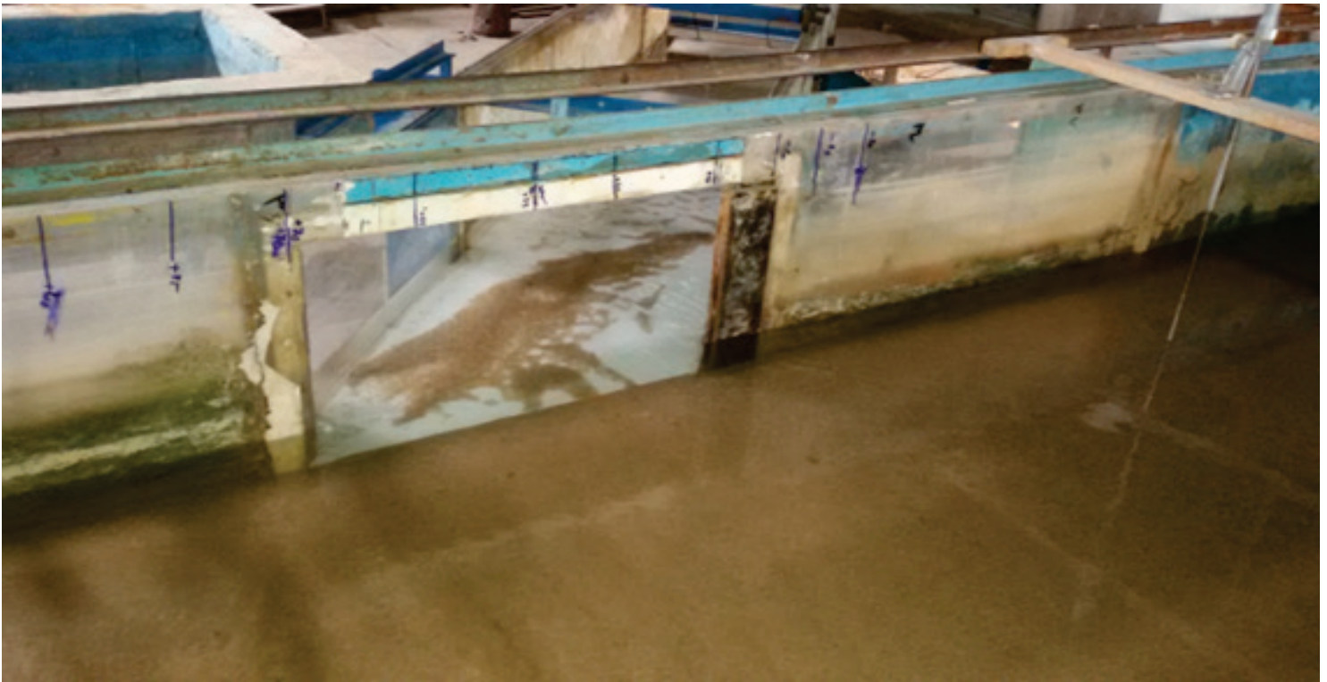
Figure 5. A view of the interior of the intake channel in the absence of the sediment control structure.
